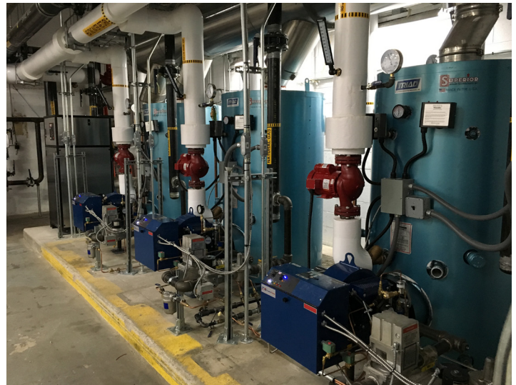
Three natural gas fired dual fuel boilers and one high efficiency boiler.
