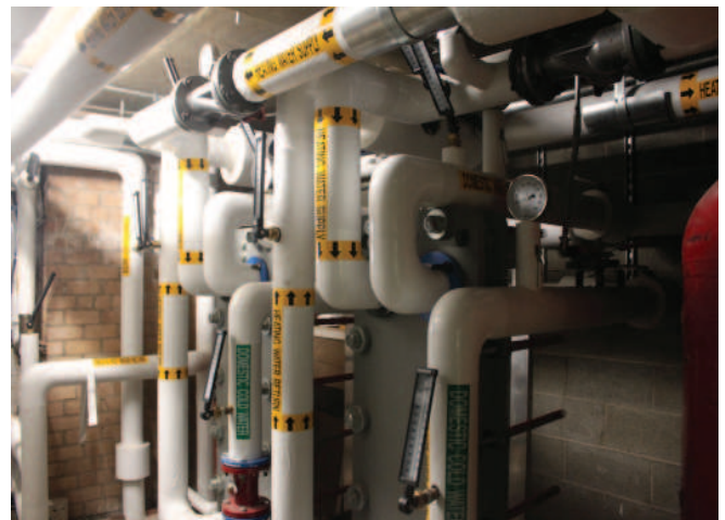
Piping and heat exchangers that generate domestic hot water.
