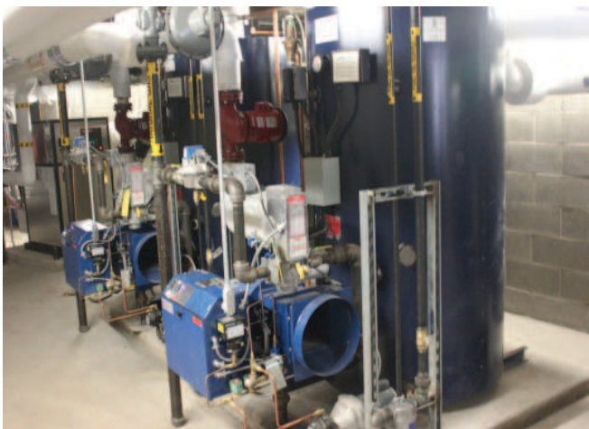
Two dual fuel boilers and one high efficiency natural gas boilers at The Windsor Suites.
